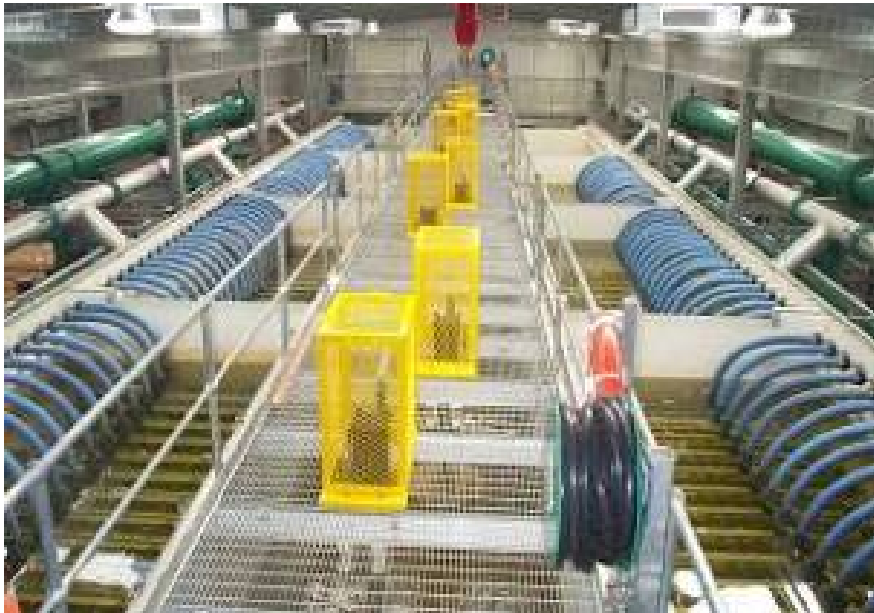
Coliban DWTP - Australia
