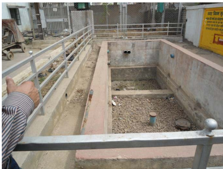
Figure 4: Recharge pit at Raipur Municipal Corporation (RMC) headquarters (Source: RMC)
