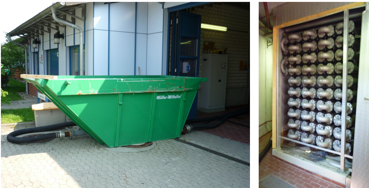
Figure 4-2: The sludge storage container (left) and the spare heat exchanger (right)
