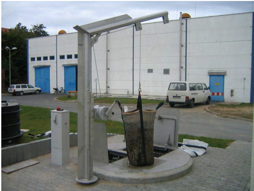
Fig. 2.4.11: Faeces dewatering facility including crane
