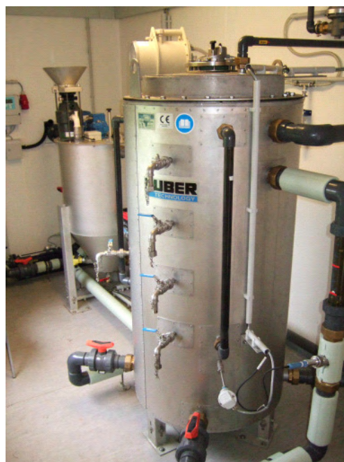
Fig. 2.4.20: Thermophile two-stage biogas plant
